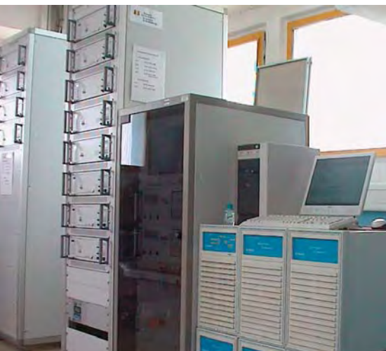
FIG 3 Equipment room with ATC system components.
