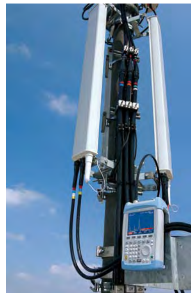
FIG 8 The R&S®FSH3, the do-it-all solution for measurements required during installation and on-site maintenance, used for measuring a mobile radio antenna.
